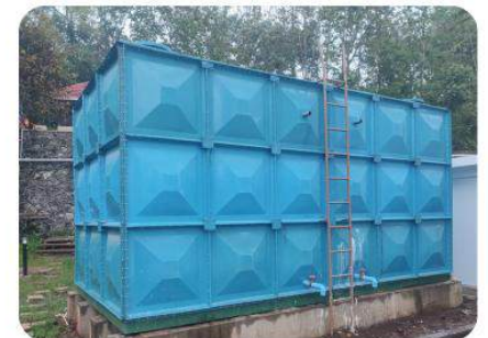
Ground Water Tank (GWT) FRP
