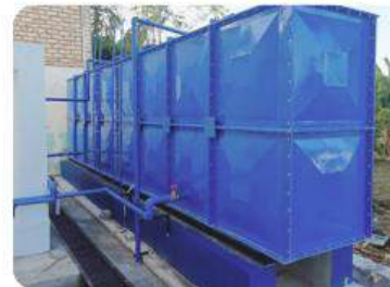
Ground Water Tank (GWT)
